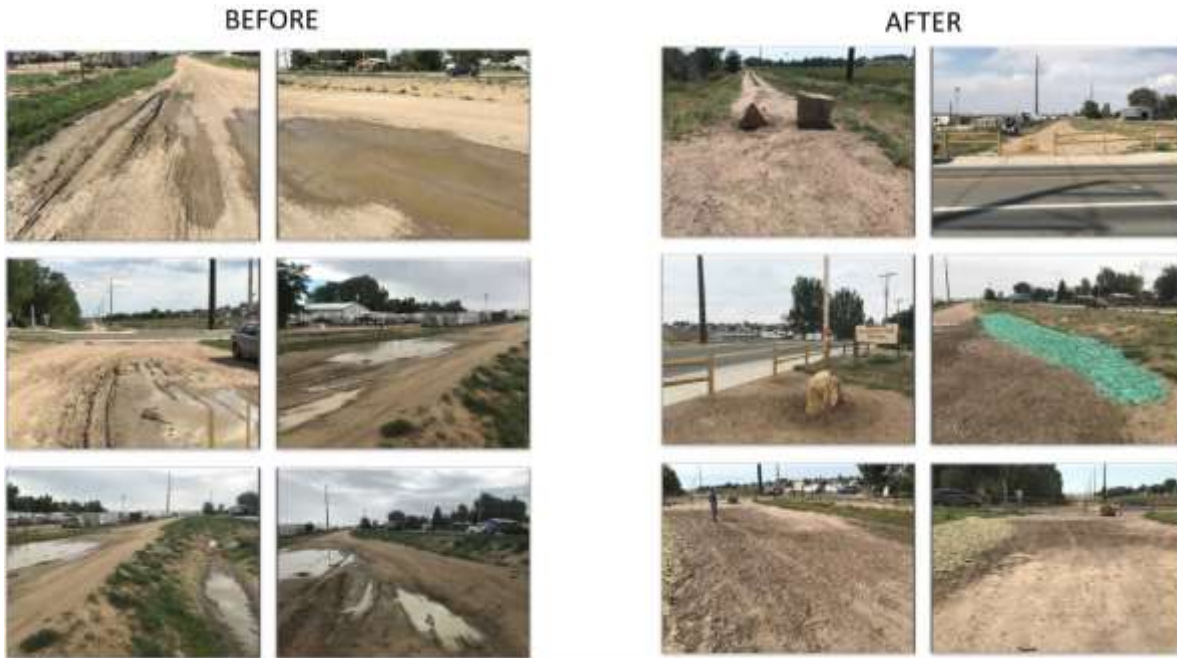
Snapshots before and after the trail access improvements along the Great Western Trail near downtown Severance
